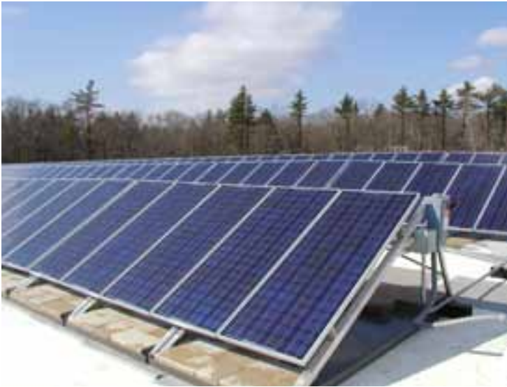
This photovoltaic array provides 150,000 kWh of electricity annually.
